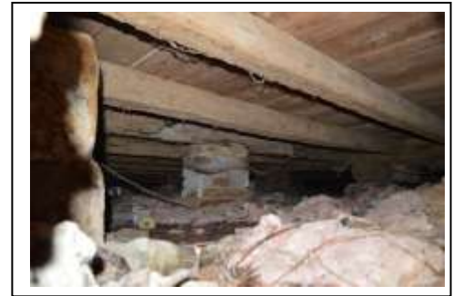
Sandstone Pier at Left, Brick at Center and Wood Log Support at Right.
